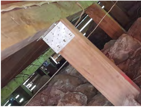
Example of anchor in wrong place.
